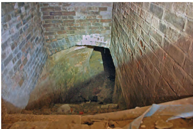
Shot through a crack in the cellar floor at number 5: stairs down to a further level
